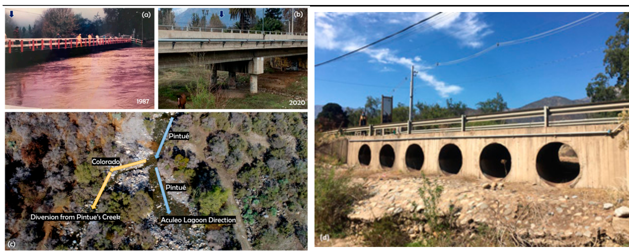
Figure A3. (a) Pintué River flows during a storm that occurred in winter of 1987 (courtesy of Joaquín Lepeley). The bridge was the measuring point for the DGA's instantaneous streamflow monitoring that occurred between 2003 and 2010; (b) A view of the current (since 2010) Pintué River flow, with a new bridge constructed by DOH (Hydraulic Works Directorate); (c) Drone-based aerial images of "Paso Godoy", one of many flow deviations at Pintué River (courtesy of Que No Muera Aculeo , an activist local organization); (d) Road crossing (bridge) at Las Cabras River (completely deviated since the mid-1990s) showing that, based on the dimensions of the hydraulic structures, significant flow rates contributed to the Aculeo aquifer during winter months (Courtesy of Marcelo Fleck).
