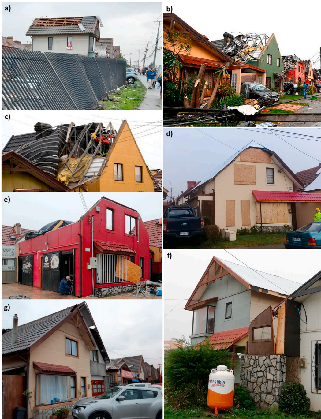
Fig. 6. Affected structures in the Brisa del Sol neighborhood. (a) Roof sheathing failure, (b) roof sheathing and joist failure, (c) roof sheathing and joist failure, (d) roof sheathing and wall opening failure, (e) complete roof failure, (f) partial wall collapse of house addition, and (g) roof deck uplift of house addition.
