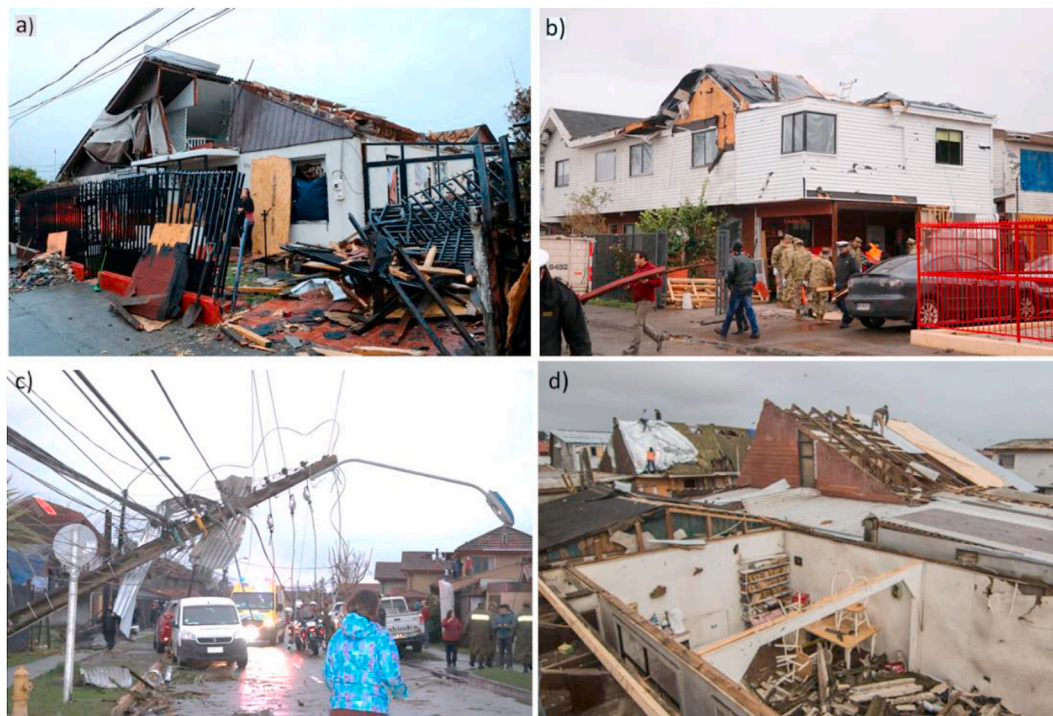
Fig. 5. Damage observed in the Salinas area. (a) Cruz del Sur neighborhood, (b) Cruz del Sur neighborhood, (c) Jaime Repullo neighborhood, and (d) Huertos Familiares neighborhood.
