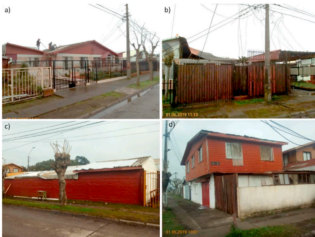
Fig. 4. Damage observed in the Higuera s area. (a) House with partial uplift of roof sheathing, (b) structure with partial roof removal, (c) house with roof sheathing failure, and (d) house with wall opening damage.
